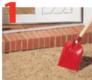
1 Excavate area large enough to fit DrainMat base, add 2" sand and compact well.
