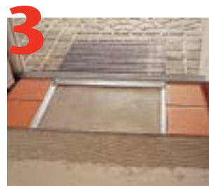
3 Install MatFrame, tile floor ensuring surface is 1/8" higher than MatFrame to prevent trip hazard.
