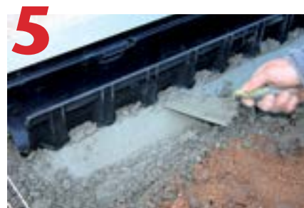
Lay 4" deep concrete bed. Lay channels working away from outlet. Concrete surround should extend up channel sides into recesses to hold channel in place.
