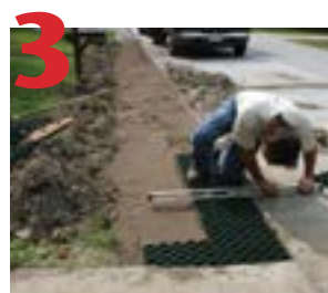
Spread sand over the bedding layer, compact well. Position GrassGrid and ensure everything is level.
